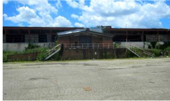
The North Exhibit Hall, above, had a collapsed roof and all windows were blown out.
